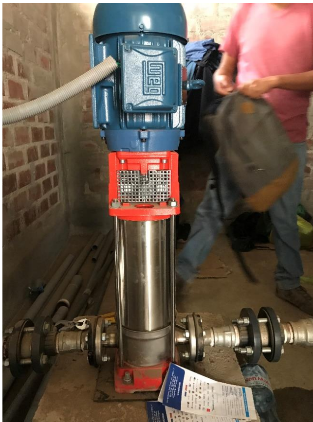
Electrobomba MULTI-V 212-FSE-T/2/6-5HP, SALMSON
